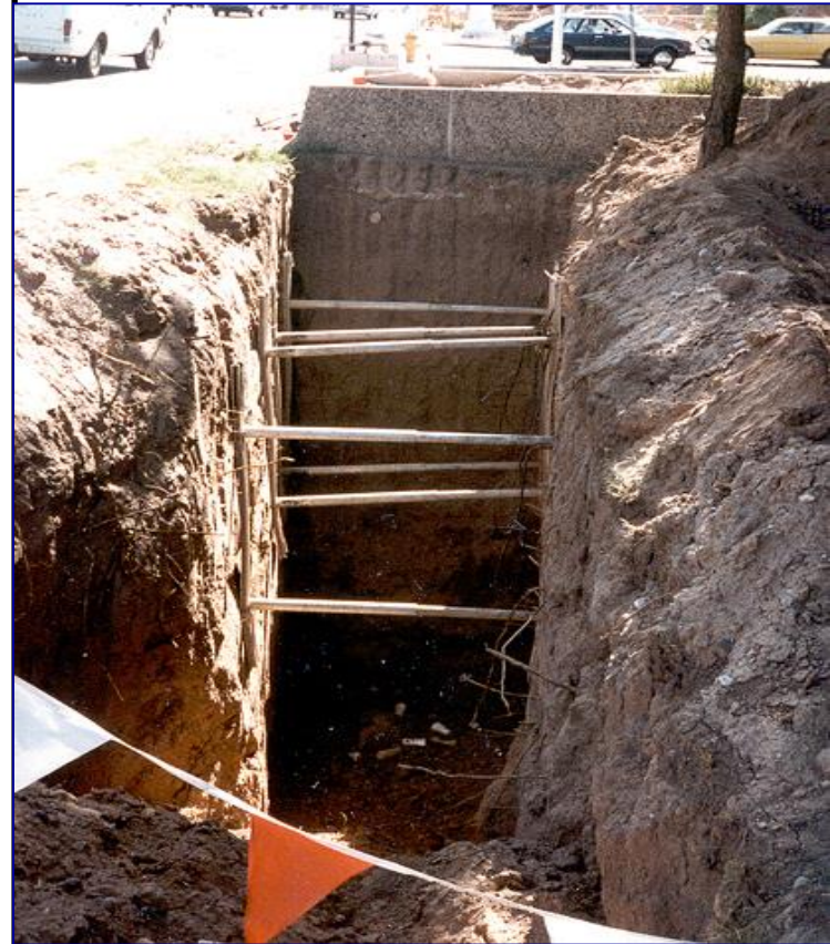
Inadequate protective system
