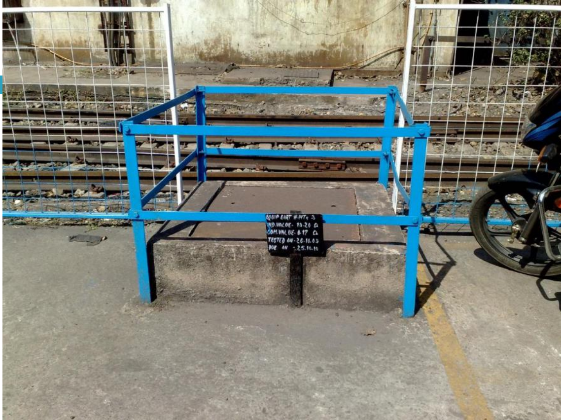
BARRICADED EARTH PIT ABOVE GROUND LEVEL
