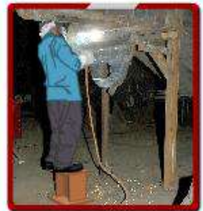
Improper Work Technique
